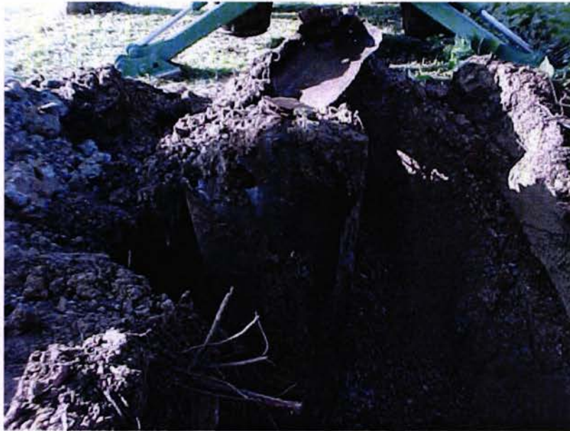
Larel Bay #1 Tank Two (full of sand)
